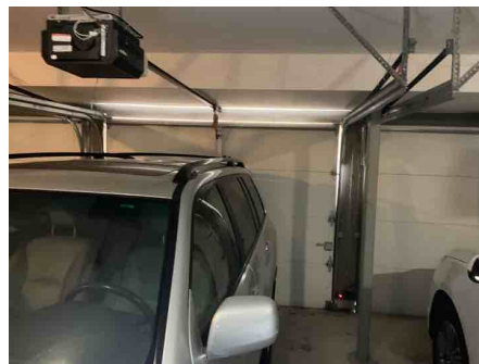
Unprotected garage doors
