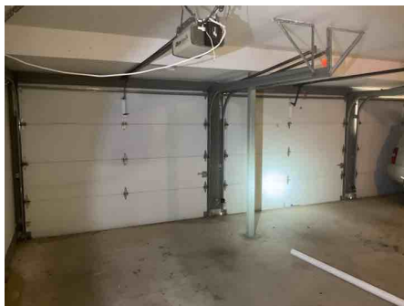
Unprotected garage doors
